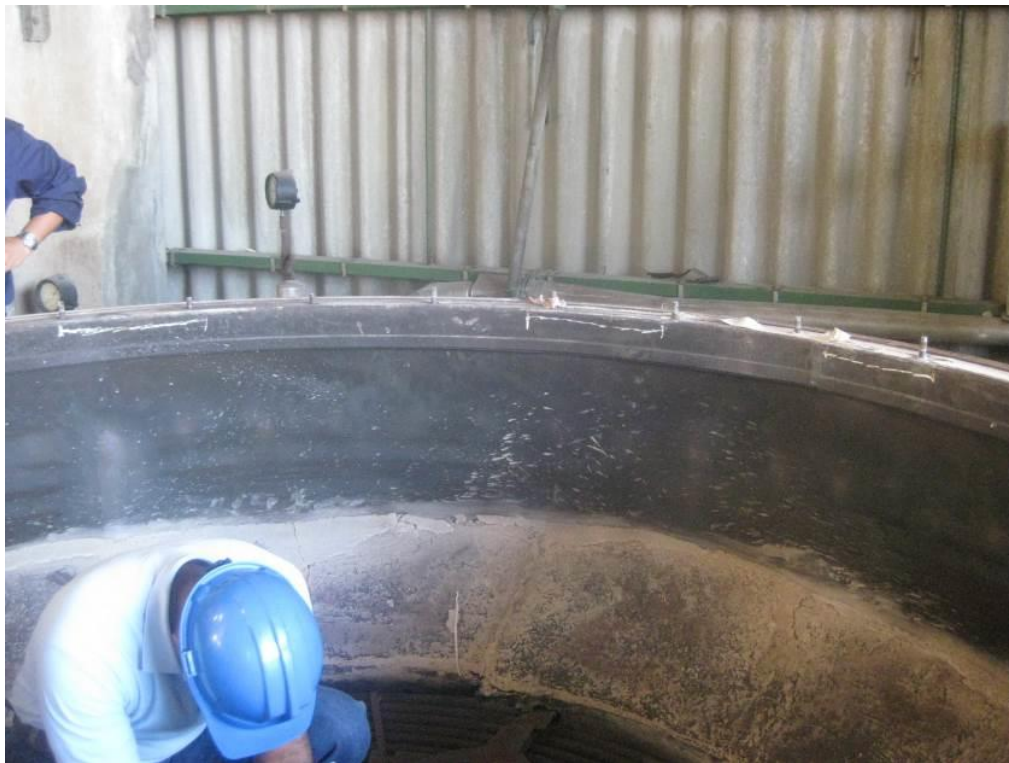
Photo 4: Internal part of the upper part of the R1101 Reactor.
