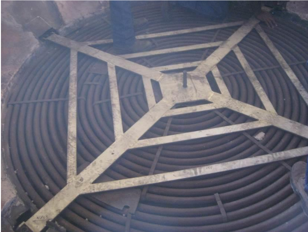
Photo 3: Support structure at the bottom of the R1101 Reactor where the Basket is supported.
